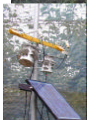
Weather sensors outside of the canopy
